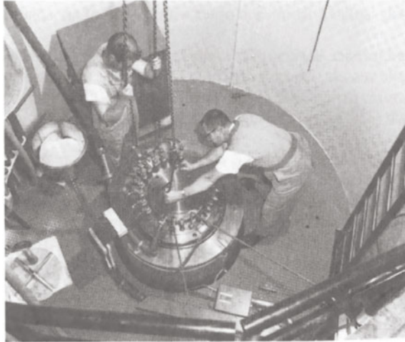
Figure 20. View of the 27-inch (68.6 cm) gas-pressure vessel within a 10-foot (3.05 m) I.D. pit.
